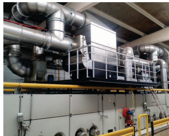
Fig. 14. Image of economizer on stenter machine
