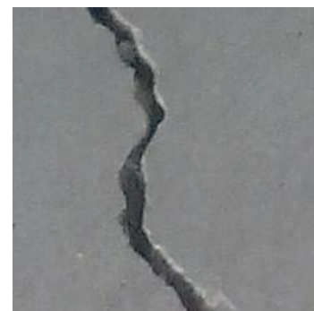
Fig. 2. Image with positive crack detection
